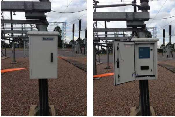
FIGURE 3: Merging Unit Installed in substation yard.
