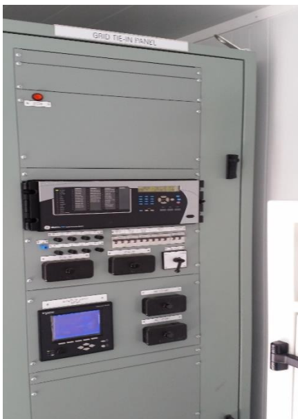
Fig. 3: Control room grid protection panel.
