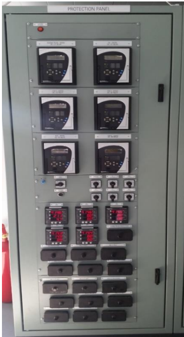
Fig. 2: Control room metering and protection cabinet.
