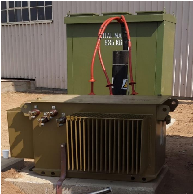
Fig.6 : Incoming RMU and 6,6 kV transformer.
