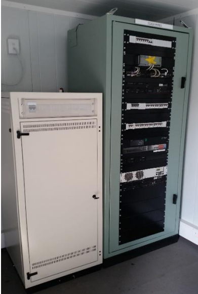
Fig. 4: Battery back up and communications panel.
